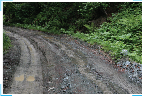
Picture 21: Curt-ruts on the road as a result of overloaded trucks driving on the road with improper drainage system and insufficient bearing capacity of pavement (Photo: Juri Beguš)
