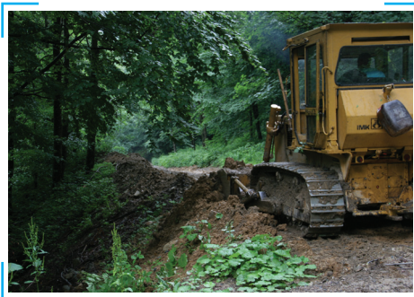
Picture 9: It is better to shape the road profile with a grader rather than bulldozer (Photo: Juri Beguš)
