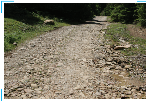
Picture 22: The lack of an upper layer is the result of poor maintenance; this road needs reconstruction (Photo: Juri Beguš)
