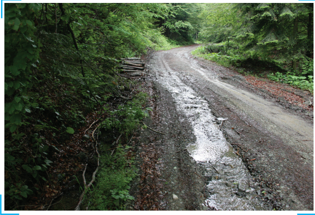
Picture 15: Obstacles in the ditch (Photo: Juri Beguš)
