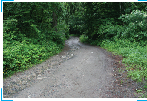
Picture 23: Overhanging branches should be removed to allow sunlight and wind to get at the road surface so it can dry out (Photo: Juri Beguš)
