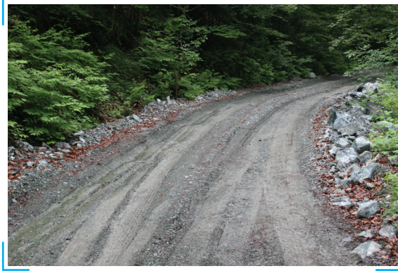
Picture 13: Avoid leaving a berm of loose material at the side of the carriageway (Photo: Juri Beguš)
