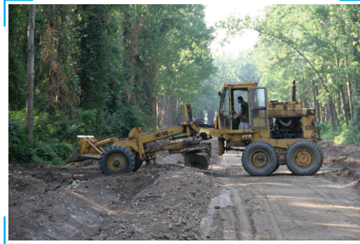
Picture 26: Graders can help achieve an appropriate shape of forest road (Photo: Juri Beguš)
