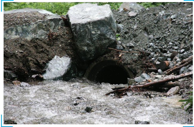
Picture 12: Culvert with an inadequate capacity (Photo: Juri Beguš)
