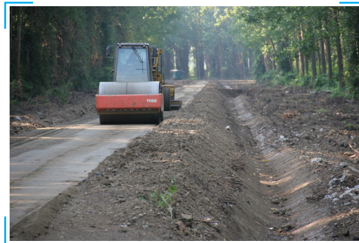
Picture 27: The final step of maintaining the carriageway is compaction. This extends the life span of forest roads (Photo: Juri Beguš)
