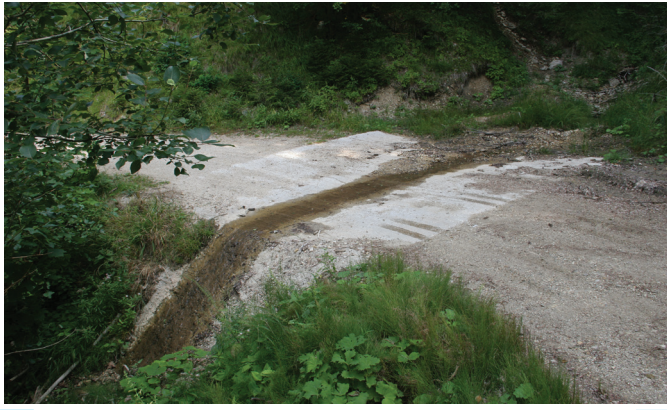
Picture 10: A concrete ford enables creek crossing over the road (Photo: Juri Beguš)
