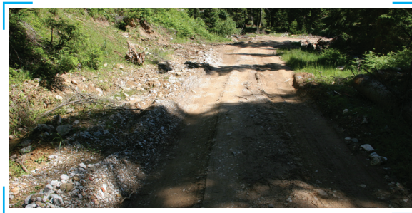
Picture 5: The lower bearing capacity of the road caused the ruts. Solutions in such cases are road closure at the time of lower bearing capacity, using proper material for reconstruction, using geotextile on the sequences of lower bearing capacity (Photo: Juri Beguš).
