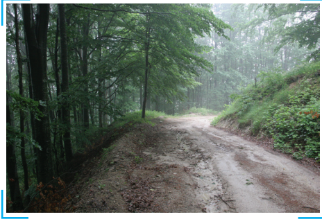
Picture 8: Heavy rain, improper use and insufficient/improper maintenance cause heavy erosion on the carriageway of a forest road (Photo: Juri Beguš)
