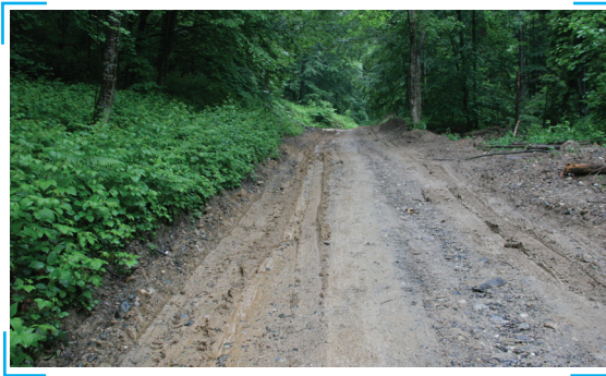
Picture 11: Surface erosion on steep ground (Photo: Juri Beguš)
