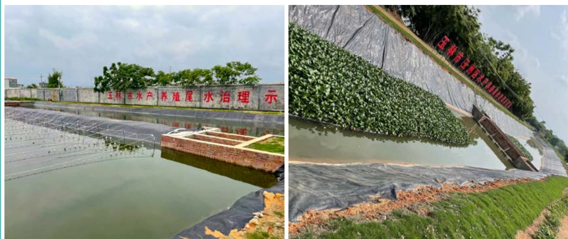
FIGURE 6.7 Aquaculture effluent/wastewater treatment facilities in the aquapark in Guangxi
