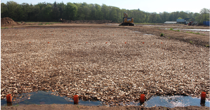
Figure 6.7 Woodchip bioreactor technology used for removal of nitrate in discharge water from an outdoor recirculation aquaculture system for trout
