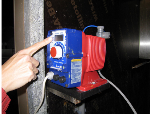
Figure 2.17 Dosage pump for pH regulation by preset dosing of NaOH. The pump can be connected to a pH sensor for fully automatic regulation of pH level
