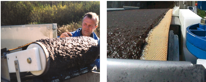
Figure 6.4 Hydrotech belt filter used as secondary water treatment for dewatering the sludge
