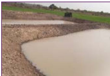
Vulnerable dyke to erosion owing to lack of cover vegetation after renovation, Guinea-Bissau, ©FAO/Mulonda Boniface.
