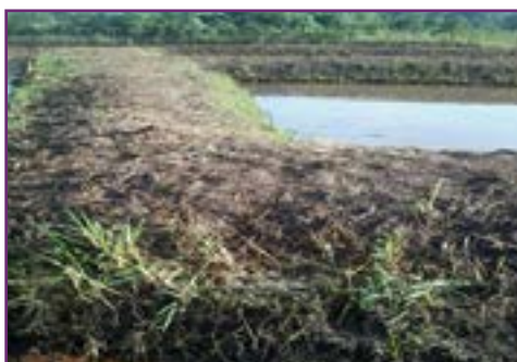
Degraded dyke, Kenya, ©FAO/Mulonda Boniface.
