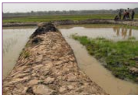
Poor dyke construction, Guinea-Bissau, ©FAO/Mulonda Boniface.
