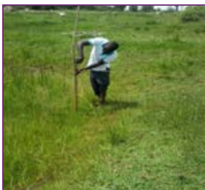
Staking out the height of a dyke for renovation, Uganda, ©FAO/Mulonda Boniface.
