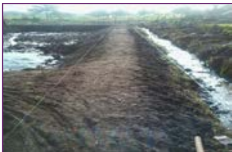
Shape pond dyke after renovation. Final shape of a dyke after renovation, Uganda, ©FAO/Mulonda Boniface.
