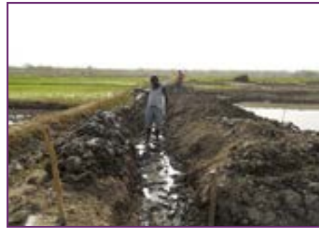
Making a core trench for reinforcing the dyke of a pond, Guinea-Bissau, ©FAO/Issa Barry.
