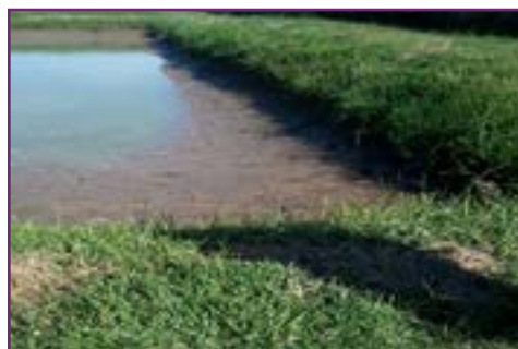
Degraded slope of the dyke, Uganda, ©FAO/Mulonda Boniface.
