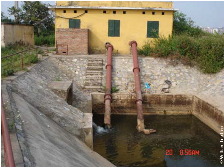
FIGURE 15: One of the electrically powered wastewater pumping stations for Bang B village from the Tor Lich River
