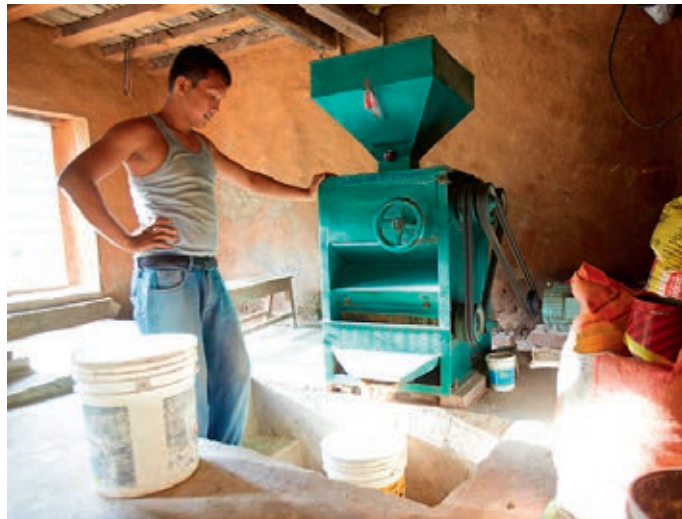
Talti village in Dhading district in Nepal: a new micro hydropower plant has made it possible to open an agro-processing plant. ©The World Bank
