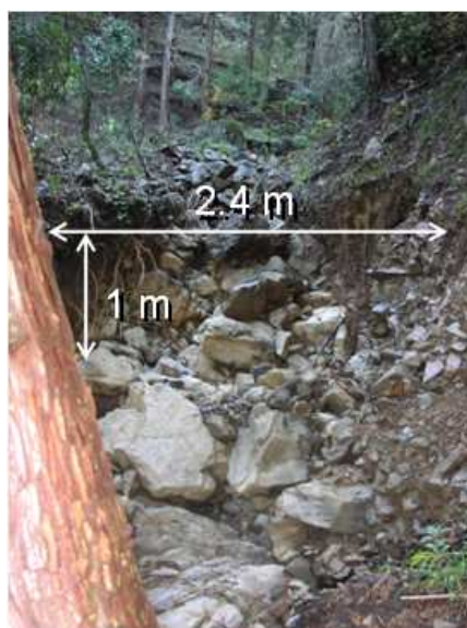
FIG. 8. Eroded truck trail after the typhoon event.
