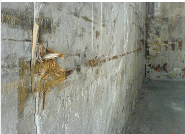
FIGURE 23 Bad bulk storage conditions
