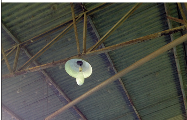
FIGURE 12 Light without protection and allowing contamination when broken
