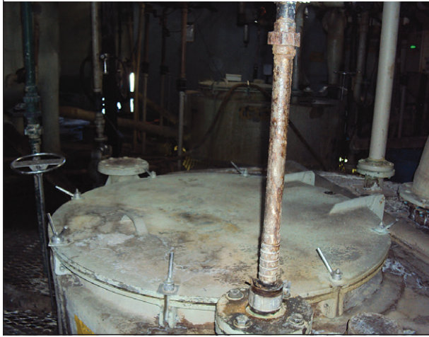
FIGURE 17 Processing equipment lacking maintenance
