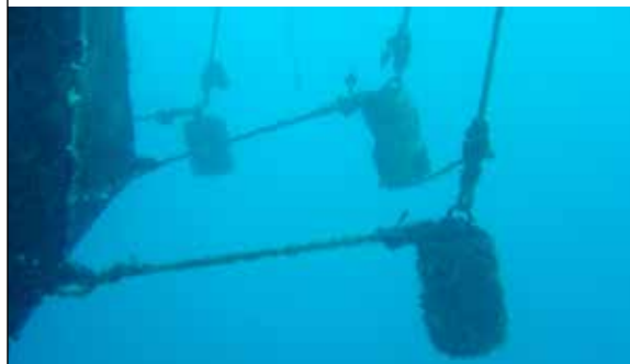
PLATE 32 Concrete sinkers installed incorrectly: the vertical sinker rope is too short and the net is hanging from the sinkers
