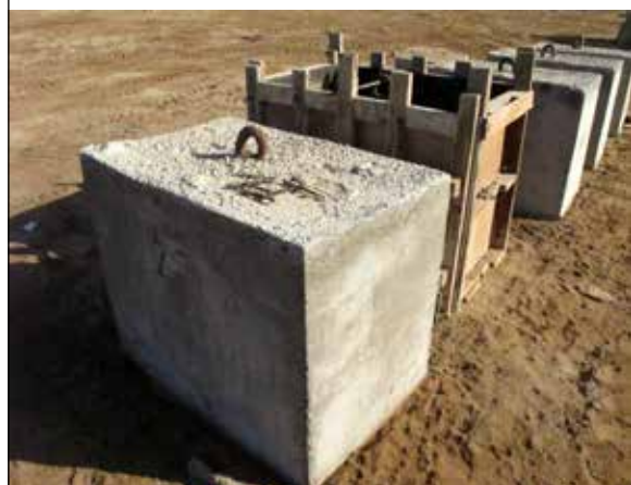
PLATE 7 Once the wooden form is filled with concrete, and the block has hardened, the form can be removed and the block left to dry for a few days
